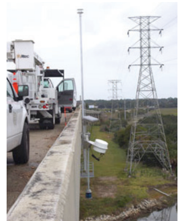
Figure 1. Florida Department of Transportation bridge wind speed monitor installation. (Source: Florida Department of Transportation)
