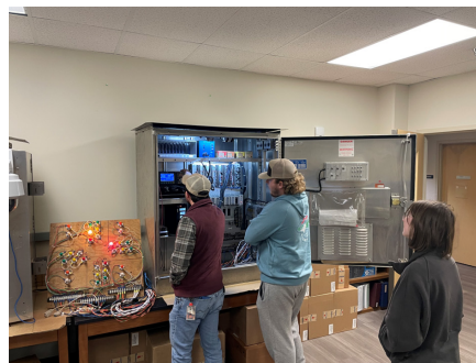
Figure 1: Student interns diagramming traffic signal phases and working with intersection light boards within the TMC's traffic signal test cabinets.
