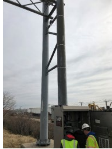
BHT South Portal Cohda RSU
